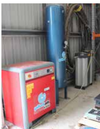
PILOT K50 AIR COMPRESSOR Receiver & Atlas Copco CD50 Drier
